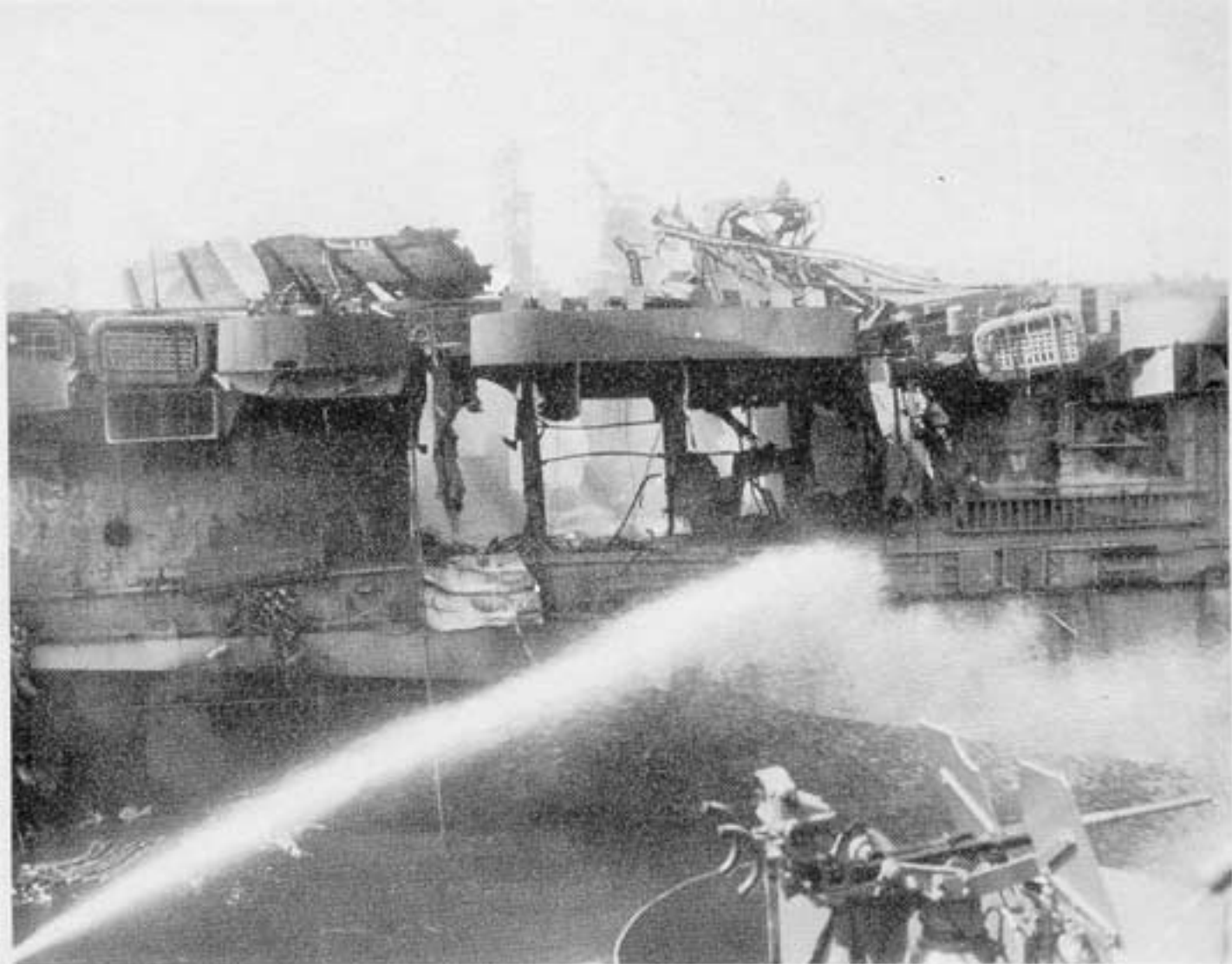
9. View of damage to port side of hangar between frames 74 and 86. Note similar damage to starboard side of hangar.
